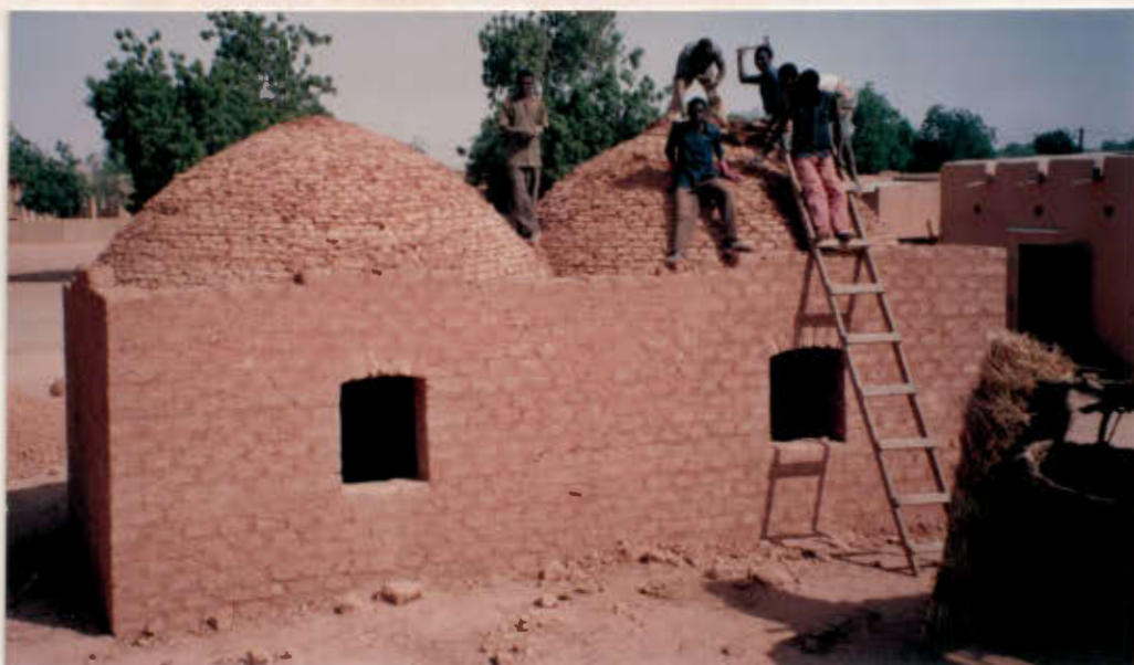
This two-roomed house with twin domes on rectangular bases is under construction during the Ouallam training programme; the design, however, is the same as that used by Mounkaila for the first owner-built and owner-funded domed house in the area.
