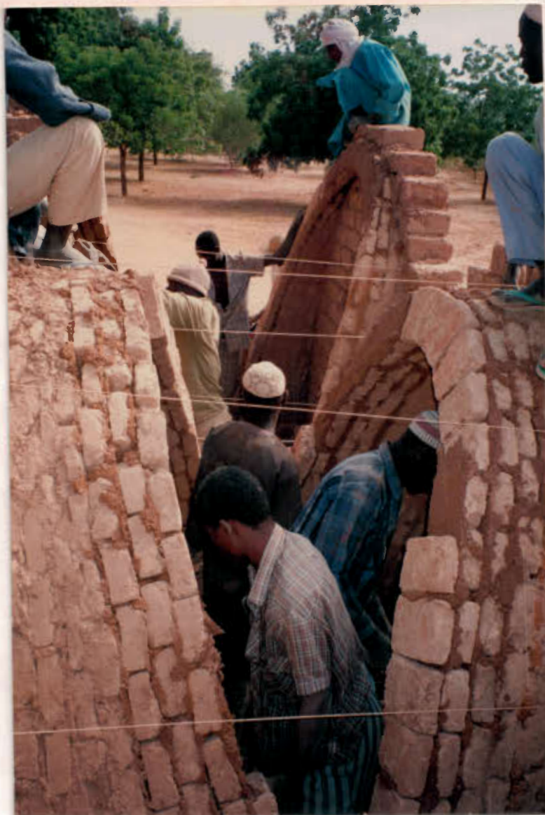
Practice work (at ground level) on vault-building during the Ouallam training programme.
