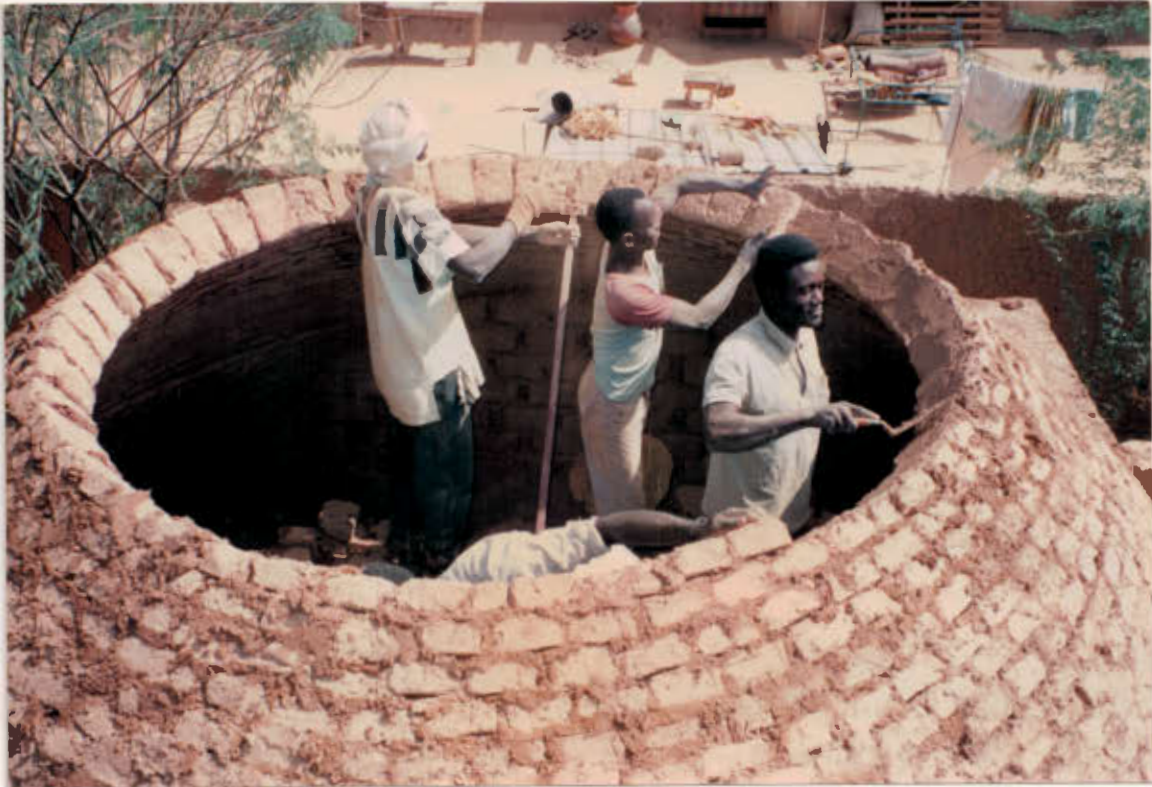
Trainees on the Ouallam training programme build a dome on a rectangular base: a radial arm shows the position and angle of each brick.
