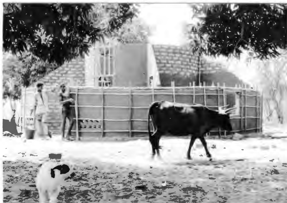
G). OUTER WALL FRAMING IN PLACE. INNER RING WALL BEING PLASTERED. (MADINA GUILLEDJI.)
