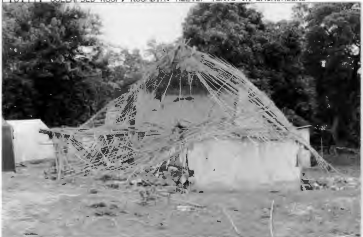
FIG.11. COLLAPSED ROOF, KOUMBIA. RELIEF TENTS IN BACKGROUND
