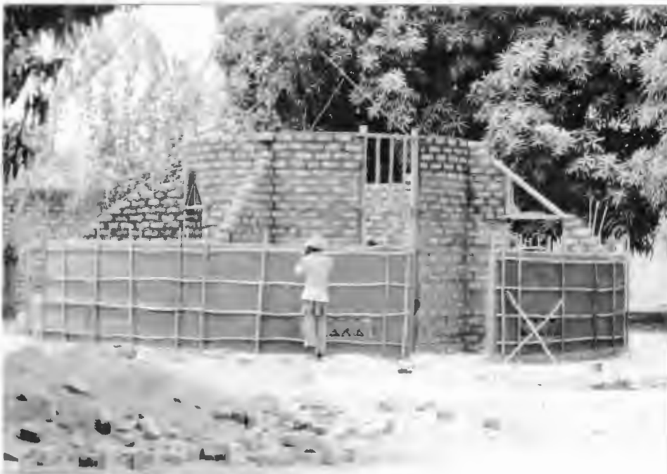
FIG. 22. OPENING IN TALL INNER WALL FRAMED UP TO TOP OF WALL - A VARIANT
