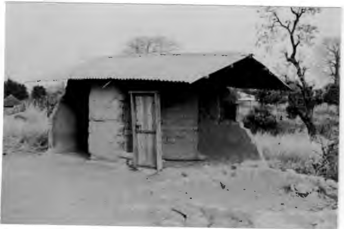
FIG. 13. COLLAPSED CORNERS ON SMALL RECTANGULAR HOUSE.
