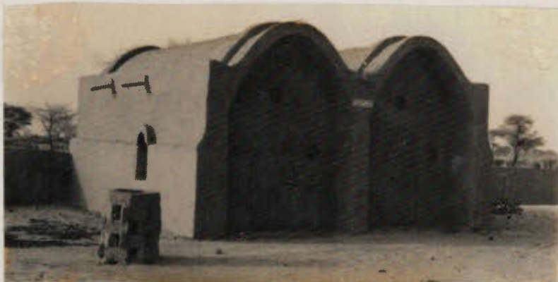
Unstabilized mud brick vaults with an earth render: after 7 years of no maintenance, structurally sound and requiring only re-rendering.
