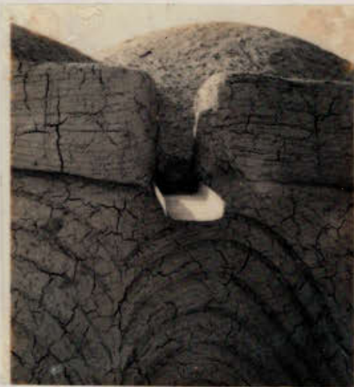
Ensuring fast rainwater runoff; using a suitable render and maintaining it regularly...
