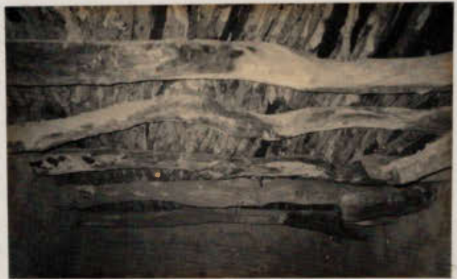
flat roof of a mud brick house - requiring enormous consumption of wood...
