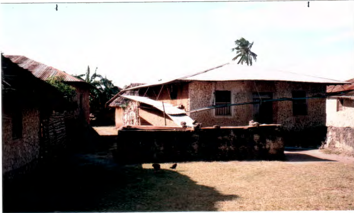
Water catchment from tin roofs, Jibondo
