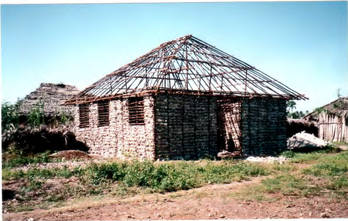
Construction Stage 1 — The wall and roof frame complete with the walls filled in with coral lumps and mortar.
