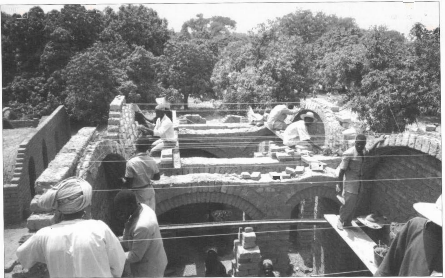
Figure 2 “Alcove” building under construction. Note the use of strings as a guide, the practice of starting the vault from both ends simultaneously, the use of off-centred vaults and open arches to create a spacious interior.
