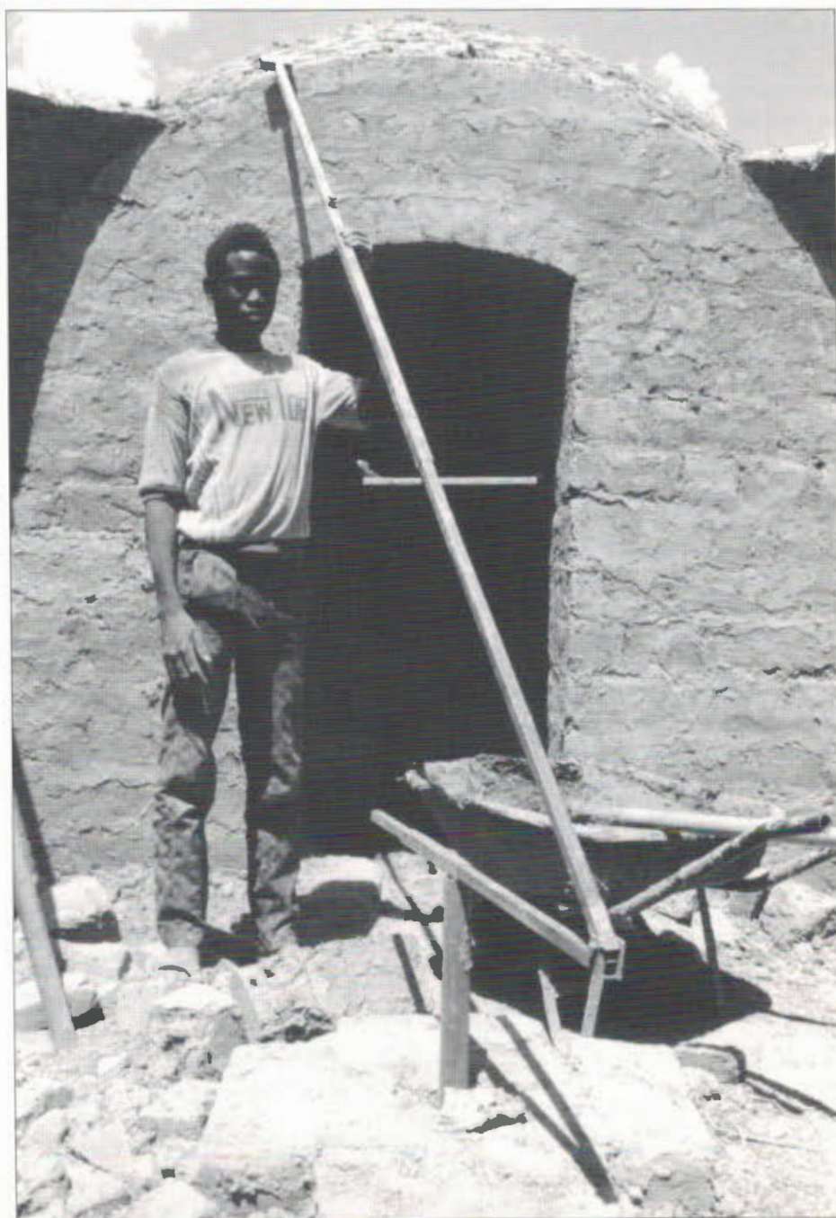
Figure 3 An adjustable radial arm is given to each mason at the end of his basic training, enabling him to build eccentric domes.
