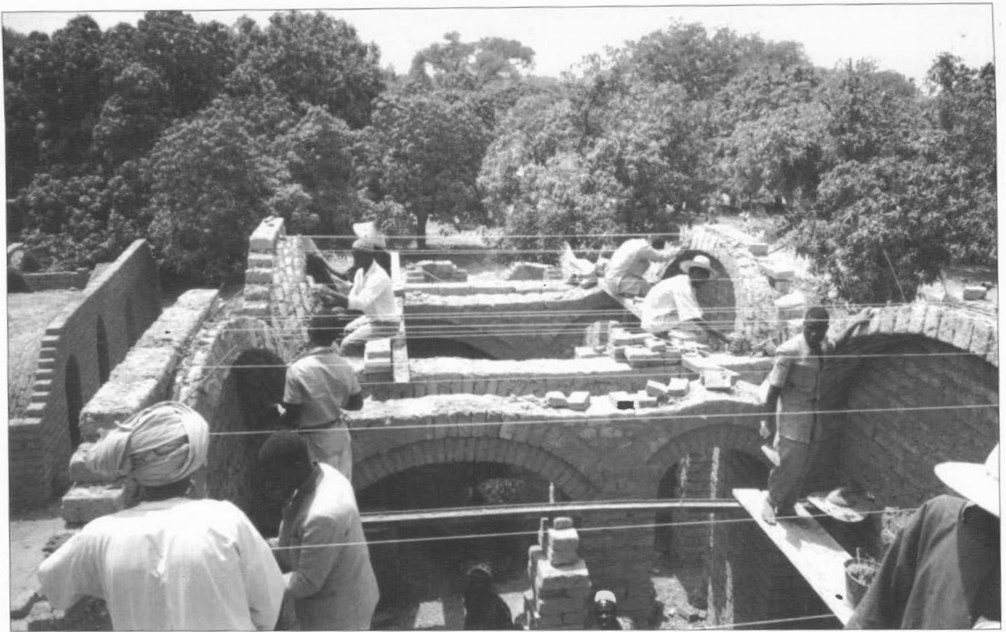
Figure 2 “Alcove” building under construction. Note the use of strings as a guide, the practice of starting the vault from both ends simultaneously, the use of off-centred vaults and open arches to create a spacious interior.
