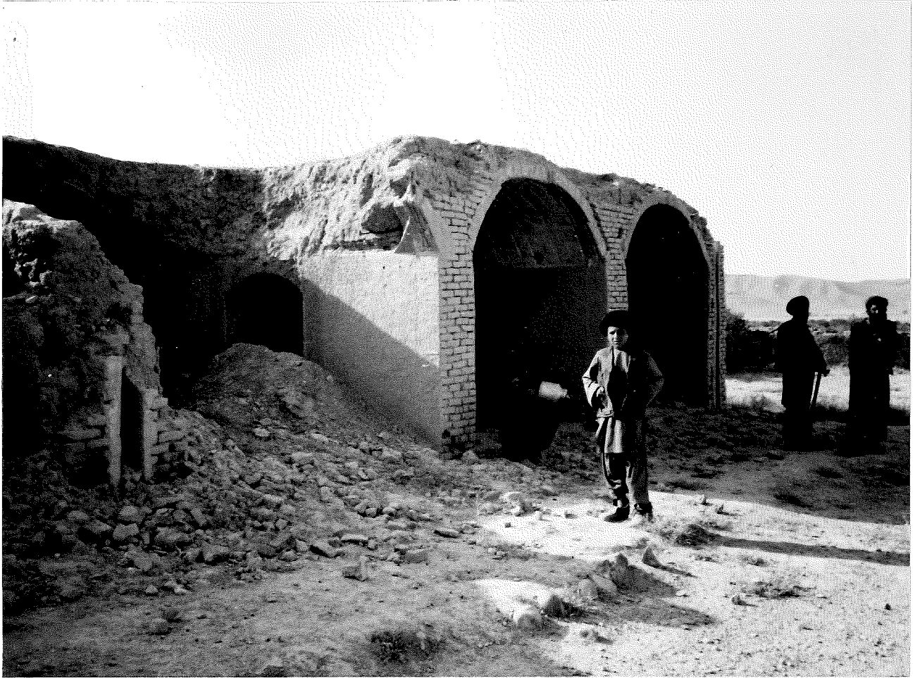
Damaged bazaar in Arghestan, Kandahar
