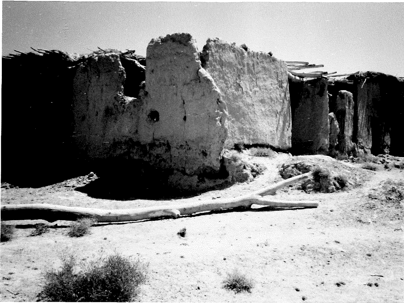
Damaged housing in Arghestan, Kandahar
